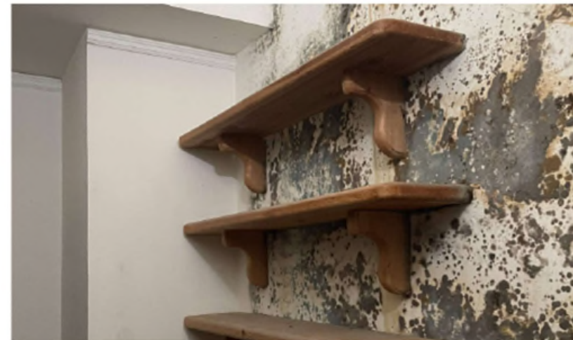
EXAMPLES OF FAILURE - INTERIOR
