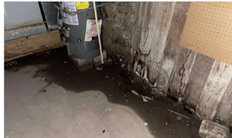
EXAMPLES OF FAILURE - INTERIOR
