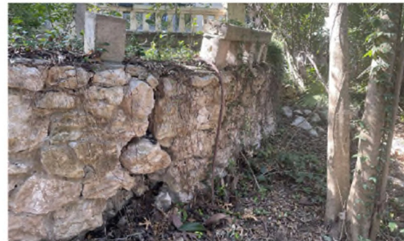
EXAMPLES OF FAILURE - EXTERIOR
